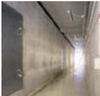
Along the 3x3 metre ventilation duct on the lower level there is a corridor providing access to the 4 silencers and the fan.
