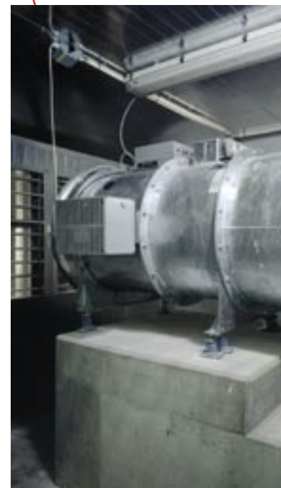
The fan (9) in the middle of the ventilation duct on the lower level has adjustable blades, and the RPM can be adjusted to control the air volume precisely from 0 m 3 /h up to 28,000 m 3 /h.
