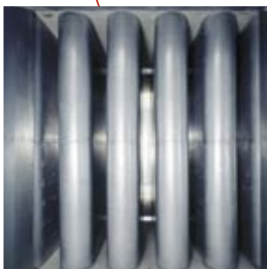
In the 3×3 metre fan duct on the lower level 2 silencers (7) have been installed on both sides of the fan (9) at a distance of 3 and 4 metres respectively. The special design and position of these silencers eliminates fan noise of all frequencies.
